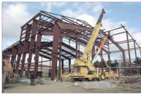
Crestview graduates Jason Smith and Beau Ray will use a crane to lift roof support beams to them to be bolted to the other framework for Crestview's Performing Arts Center. Operating the crane is another Crestview graduate, Bob Hoop.
